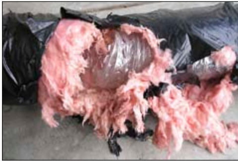
An example of the damage to the Danner's heating ducts
