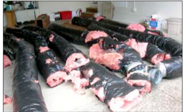
The raccoons destroyed or damaged all of their HVAC ducts
